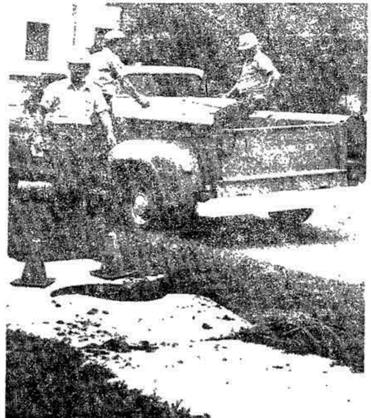
LIMA SEWER Division workers stand by a blasted out manhole on Jefferson Street Tuesday afternoon following a series of explosions caused by fumes from about 5,000 gallons of gasoline that leaked into the city sewer system. The source of the gas spill was traced to the Ford Motor Co. engine plant at Bible Road and Sugar Street in Bath Township. No serious injuries were reported. (News photo by Dennis Laman)
